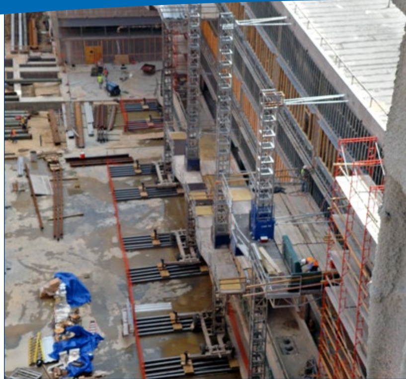
16 units involved in the re-development of the San Antonio, Texas Veterans Hospital.
