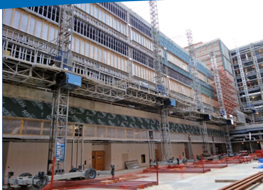
A variety of trades, including masons and framers, utilized the KPM-8 mast climbers.
